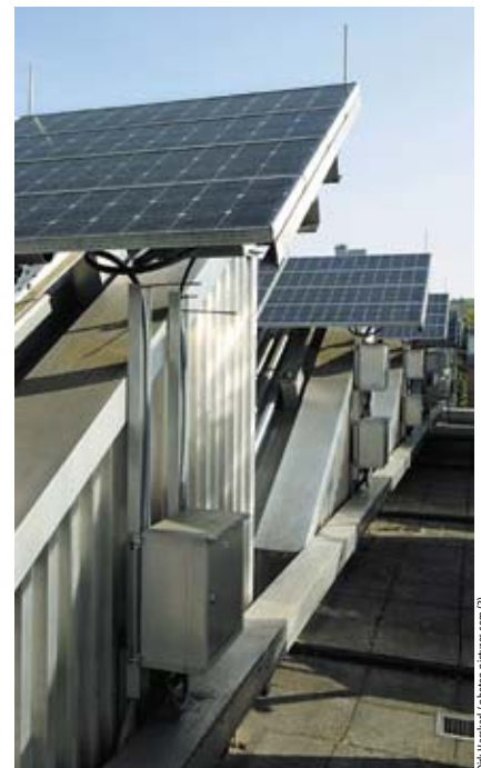
Fresh air: The in-house system on the roof of the school is just one of many to have its work logged by the PV lab.
